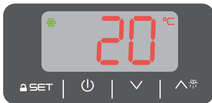
panel encendido control panel on
